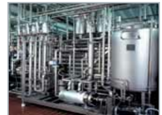
GEA TDS UHT Plant
